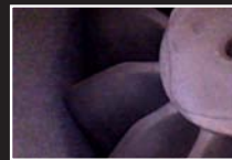
Exhaust fan blades using 6mm Long Focus camera (VSA2-1)
