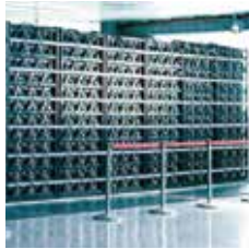
Energy storage system
